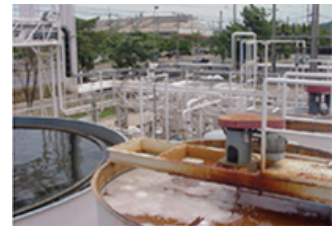
General effluent treatment facilities
