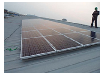
Photovoltaic power generation panels
